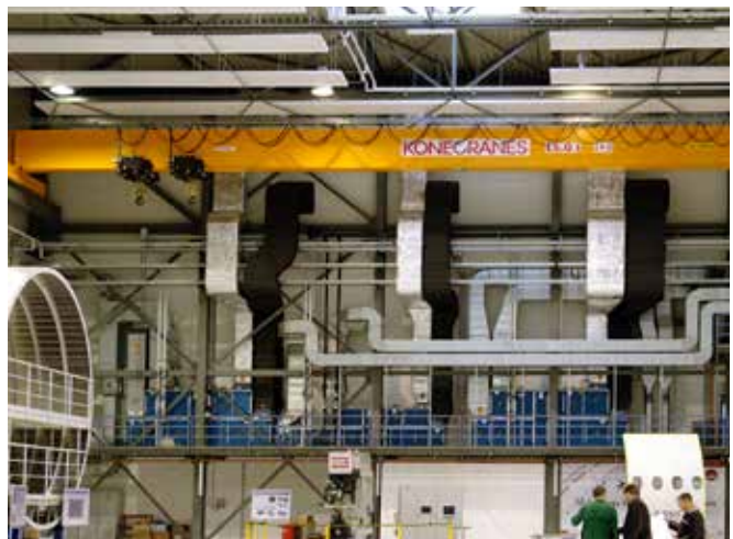
Technology Center Nordenham
