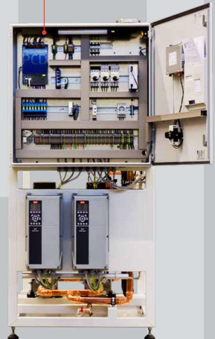
Fig. Right: Redundant hydraulic station etaHydro with frequency converters and Saia DDC (Project Agalpesion ev. KH, Giessen)
